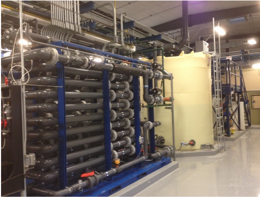
Figure CS4-1. HiPOx advanced oxidation treatment system.
